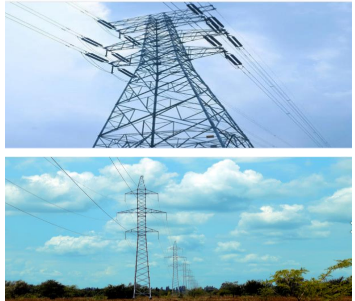
Figure 2. 220kV Double circuit transmission tower and line [33,34]
